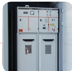
Substation high voltage chamber
