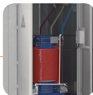
Substation transformer room
